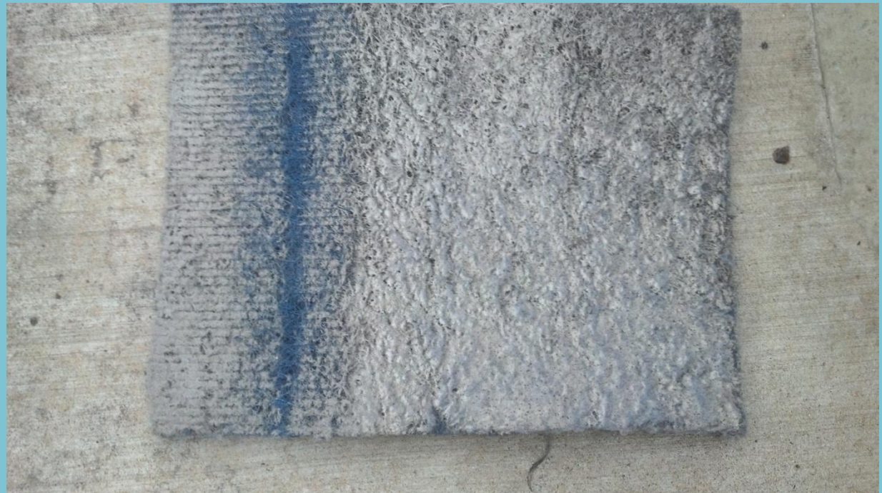
Plugged Furnace Filter discovered at UUI!
